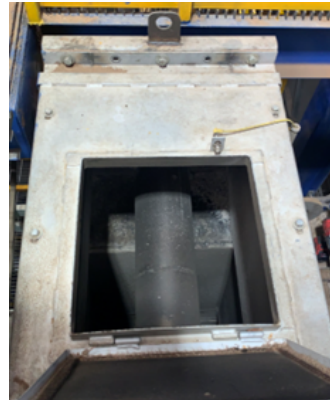
Picture 1 – view into the hatch on day 2 after the furnace burned out
