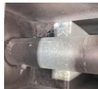
Picture 2 – view onto the ledge on day 2 after the furnace burned out
