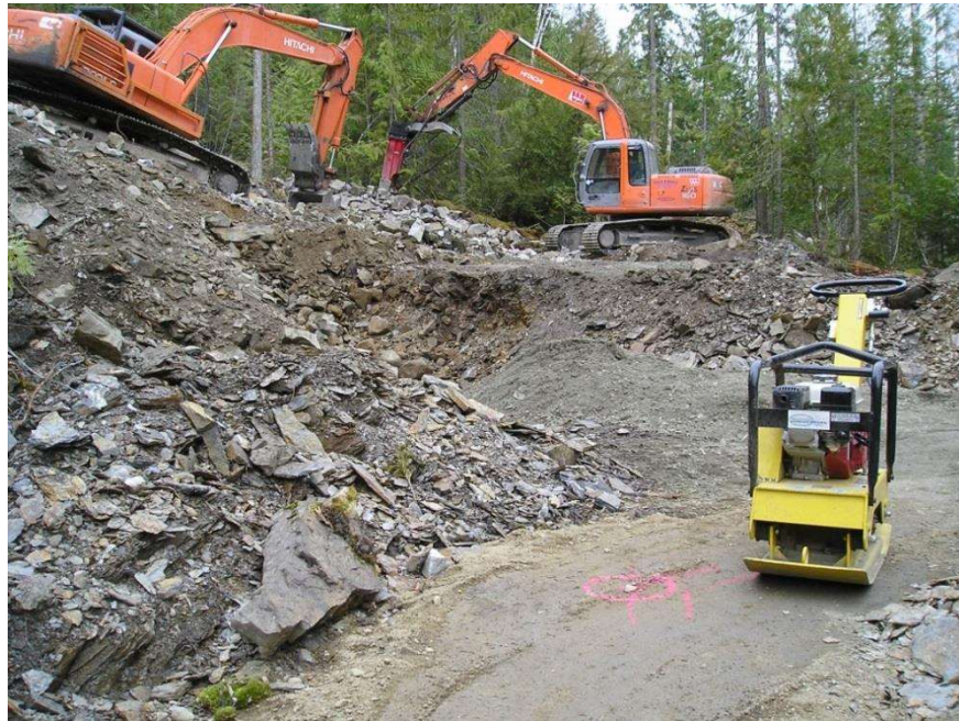
Preparing future home site for footings near Shuswap Lake, BC. Source: Chris Cole, P. Eng.
