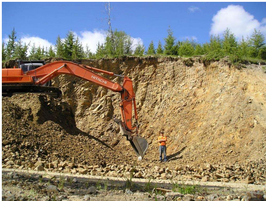
Borrow Pit Development for Road Re-surfacing Project. Source: Chris Cole, P. Eng.
