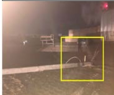
Power Pole after struck by machine
