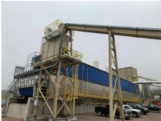
A view of the bed dryer infeed at Pinnacle's Williams Lake, B.C., plant, showing the infeed conveyor and metering bin supplied by Continental Conveyors. Photo courtesy Pinnacle Renewable Energy
