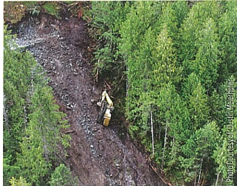
Significant construction initiated slide event on BC's coast involving road construction on a moderate to moderately steep slope through a wet draw containing organics over compact sandy-clay soils.
